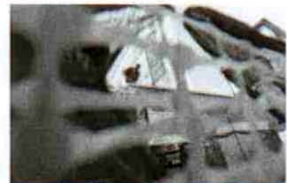
GOING UP: Construction work in the Johannesburg CBD — 22percent of Sanyati Holdings' projects are now in Gauteng Picture: Moeketsi Moticoe
