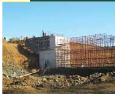
Construction of bridge as part of the R102 road upgrade (Mt Edgecombe)
