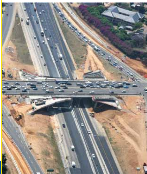
The widening of the William Nicol bridge over the N1 freeway, Bryanston
